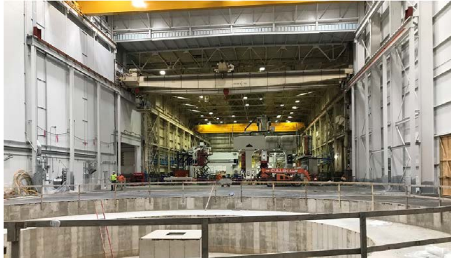
Figure 3. New IMT factory assembly building with concrete pier foundation for the azimuth bearing assembly.
