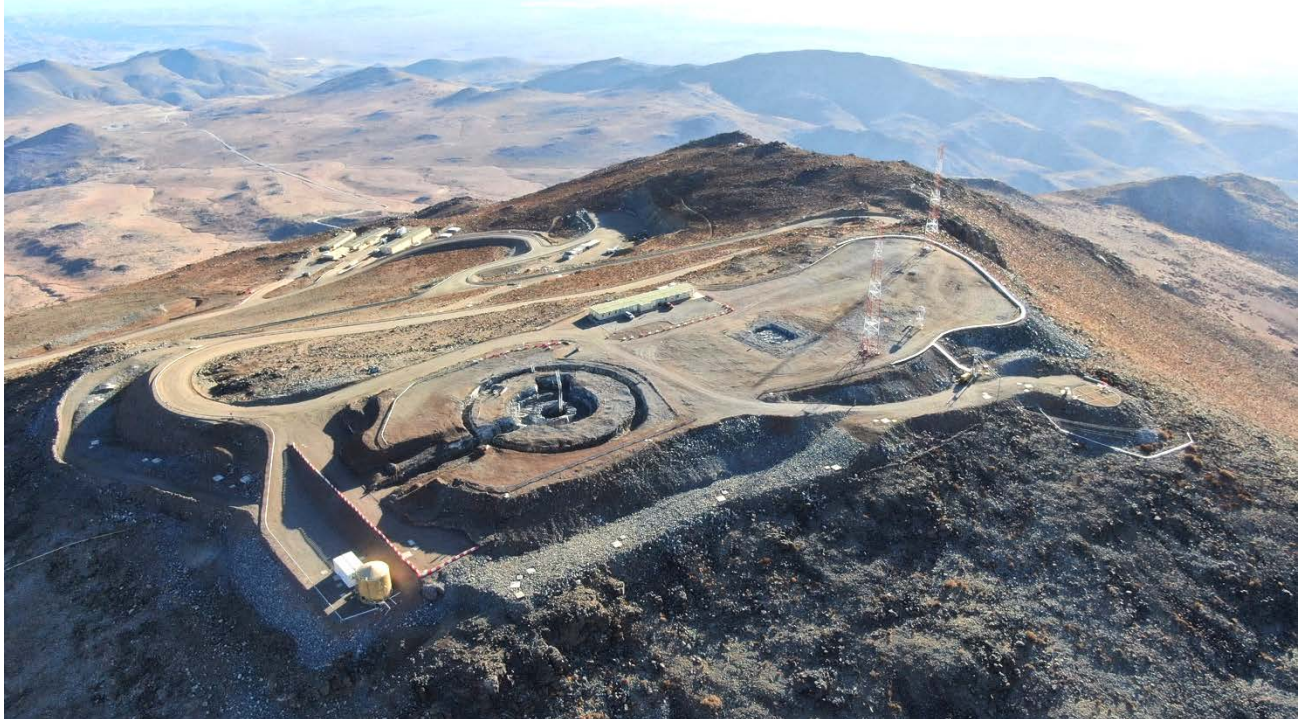
Figure 22. The GMT site following completion of hard rock excavation and utility distribution construction packages.
