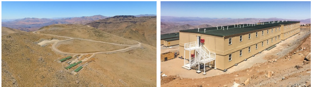
Figure 14. Left: Support site no. 2 showing residence, dining and recreation facilities ready to support construction. The leveled summit site can be seen above support site no. 2. Right: Construction workers' residence accommodates a crew of 200.
